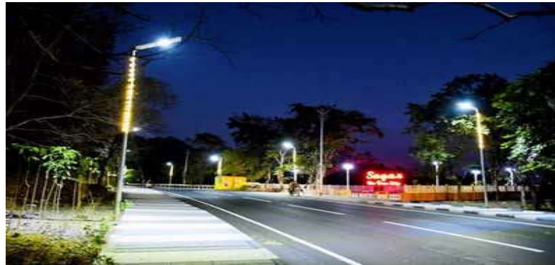
Fig. 8. Sensor-controlled LED street lighting on an arterial road in Sagar Smart City.
